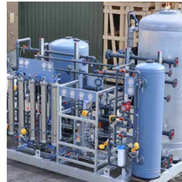
WATER PURIFICATION PLANT FOR QUALITY PURE WATER
